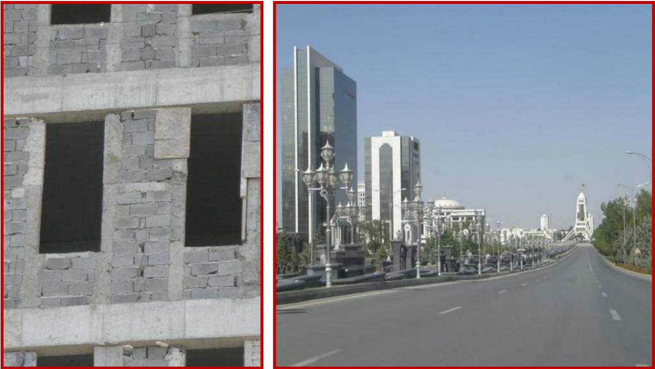
Picture 11 (left): Since all new buildings are covered with thin layers of white marble, insufficient workmanship is concealed for a while. But buildings erected only a few years ago already show clear signs of degeneration. Given Ashgabat’s location in an active earthquake zone, the outcomes of an earthquake could be disastrous. The picture shows a ministry in southern Ashgabat days before being covered in marble (April 2009). Picture 12 (right): Road with several banks and ministries in central Ashgabat (September 2009).
